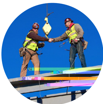
"Topping out" ceremony at Kenai Peninsula College's (KPC) Career and Tech Center.
